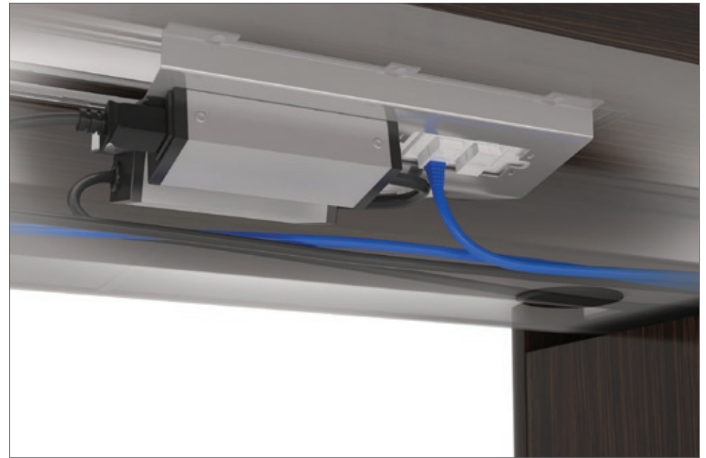
Cable management from PowerData Module
